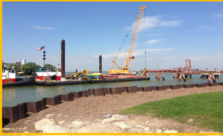
Removal of old dredging pipe on the mouth of the Fox River
