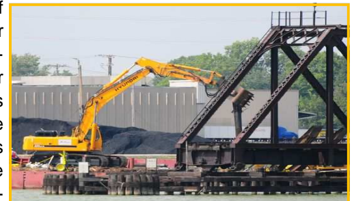
Workers remove pilings on Monday, September 14, 2014 while tearing down the Porlier Street railroad bridge over the Fox River in Green Bay (Photo: H. Marc Larson/Press-Gazette Media/@HMarcLarson)
