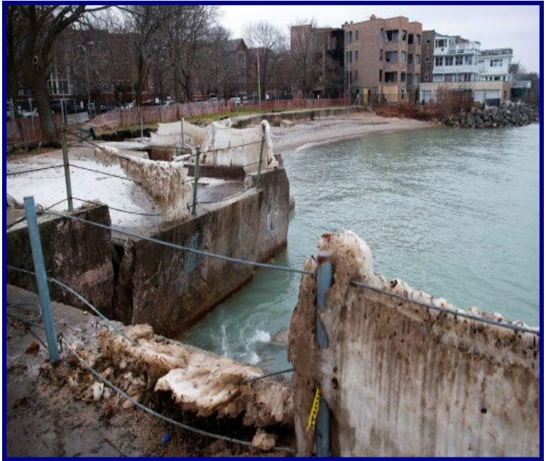
High water levels in Lake Michigan erode a walkway and seawall (Credit: Scott Olson/Getty Images)
