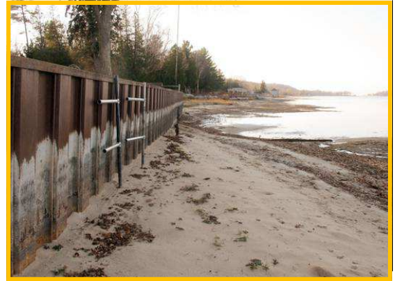
In this Nov. 2012 photo, white streaks on a steel breakwall show the normal water level on Portage Lake at Onekama, Mich., which is connected by a channel to Lake Michigan. Two of the five Great Lakes – Michigan and Huron – are at their lowest level on record. Photo taken by John Flesher
